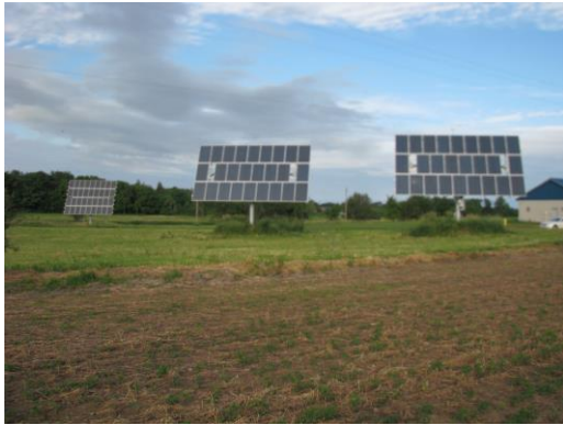
10 kW Tracker Solar Systems Seaforth Water Plant
